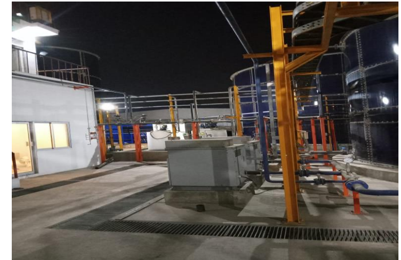
Equalization Tank blowers
