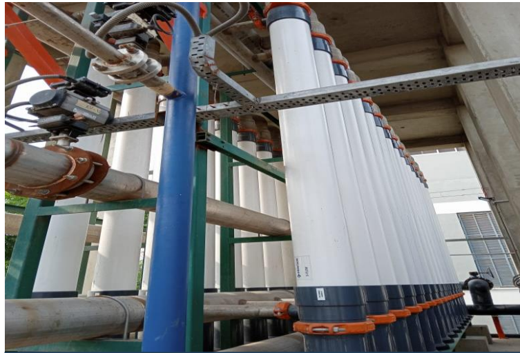
MBR (Membrane Bio Reactor)
