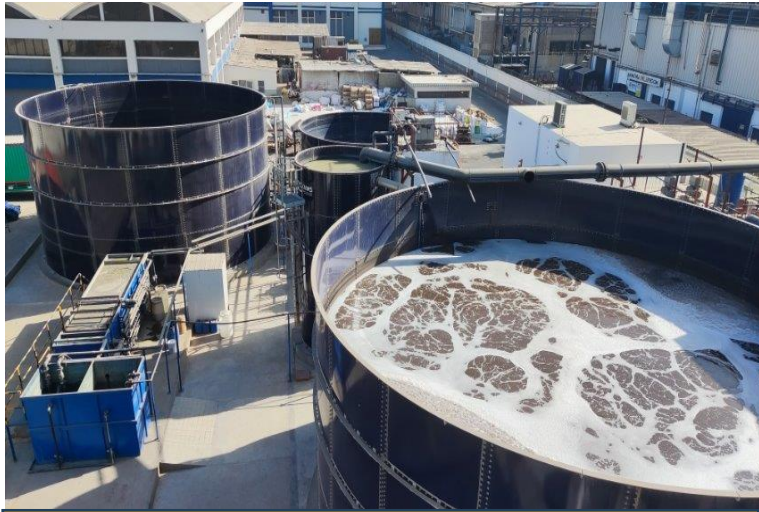
BRT (Bio Reactor Tank) buffer tank
